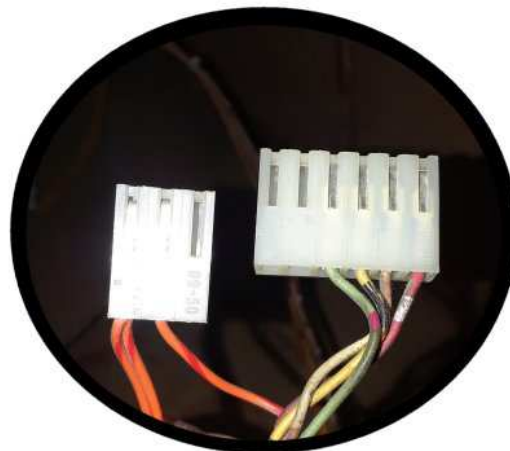
Photo: 3 and 6 pin video signal connectors disconnected.
