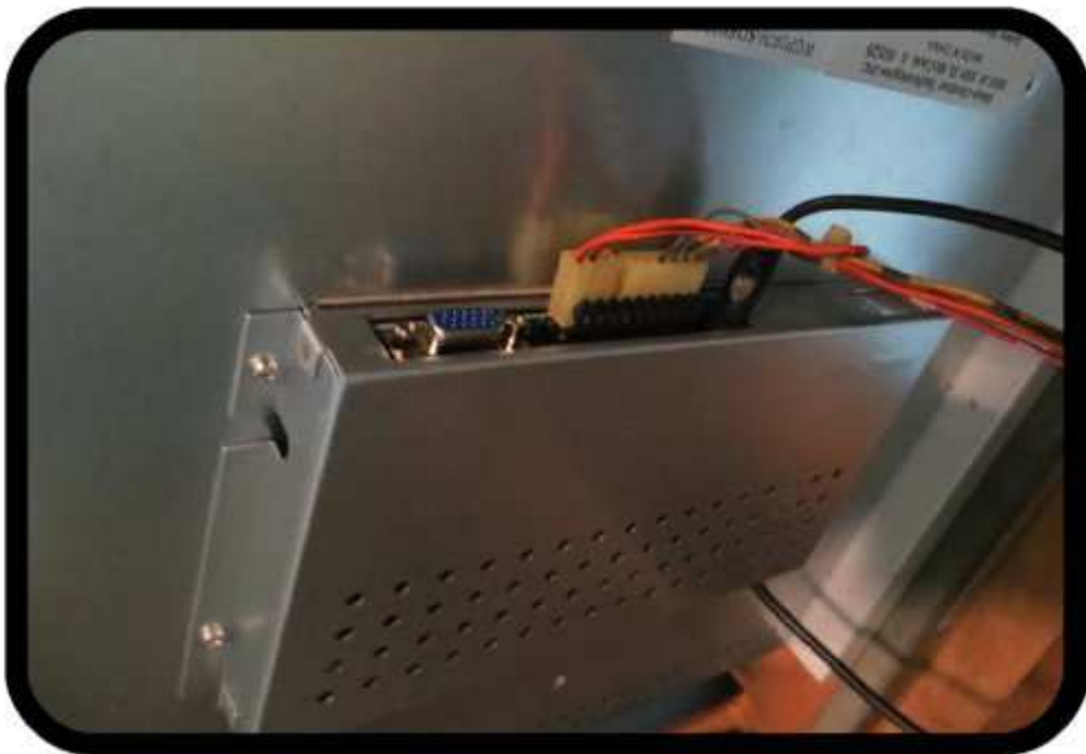
Video signal and Power connections
